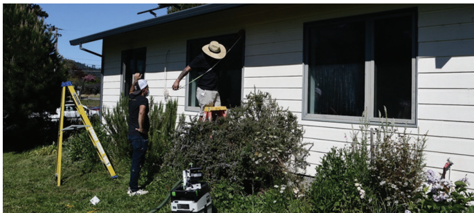
New windows being installed at the CLAM "Yellow House" on Highway One. Photo: Shauna May Photography
